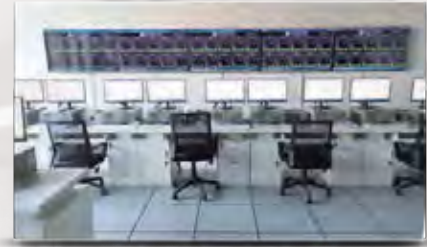
Large Screen Data Monitoring System
